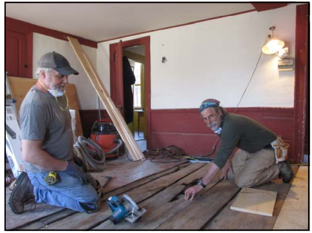
Tom Gasser and John Armstrong laying floorboards in the Strong-Howard House Keeping Room Photo by Christina Vida
