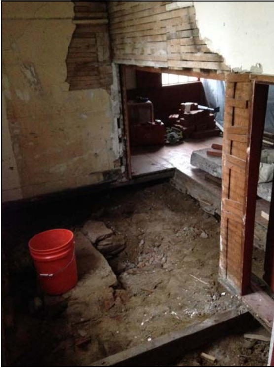
The 1954 chimney and fireplace came down in late 2014. Photo by Christina Vida
