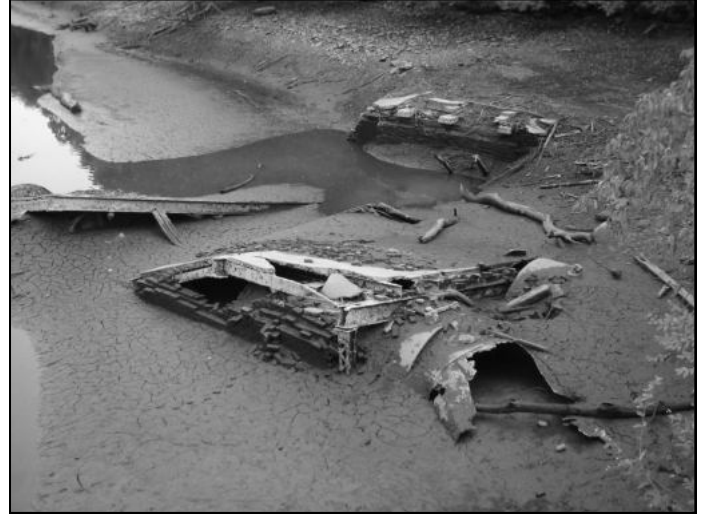
Photo 4: Penstock Remains, 2010 Photograph by the author, 2010.58.33
