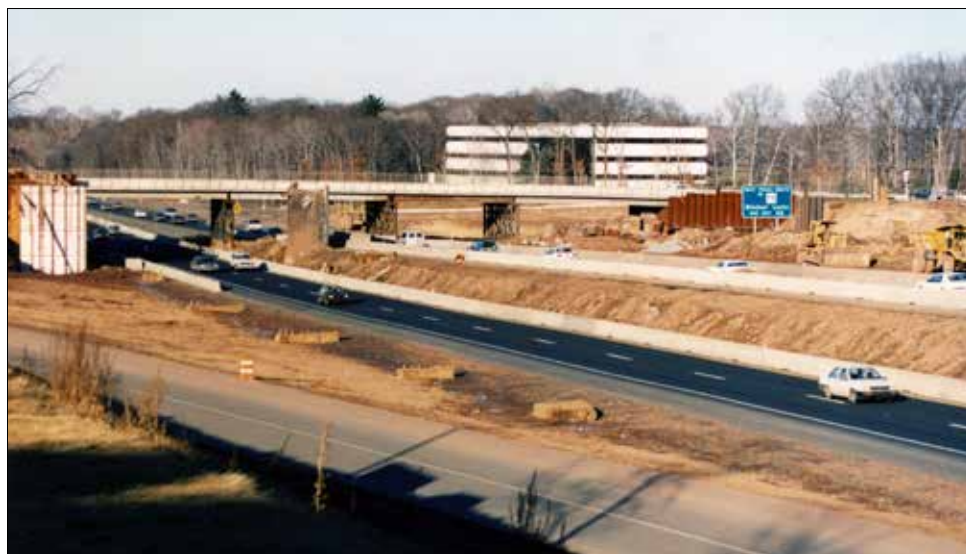
Construction underway along I-91 and the Bloomfield Avenue overpass in 1990. HOV lanes and their associated on/off ramps, which were added between the already existing highway lanes, were one of the most contentious elements of the I-91 expansion plan. | WHS collections 1992.42.R35-24A. Photo by Adelbert Coe.
