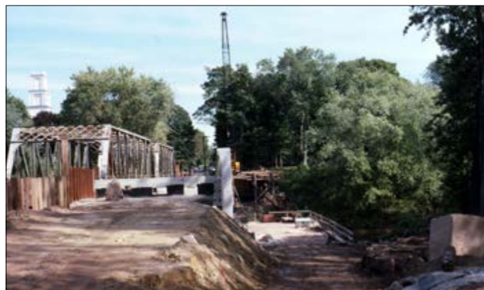
1989. In September of 1989, construction began on the current bridge over the Farmington River, placed in the same spot where the trolley bridge used to be. WHS collections 1992.42.41.443. Photo by Adelbert Coe.
